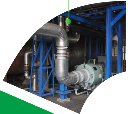
▽ Steam turbine and biomass boiler
